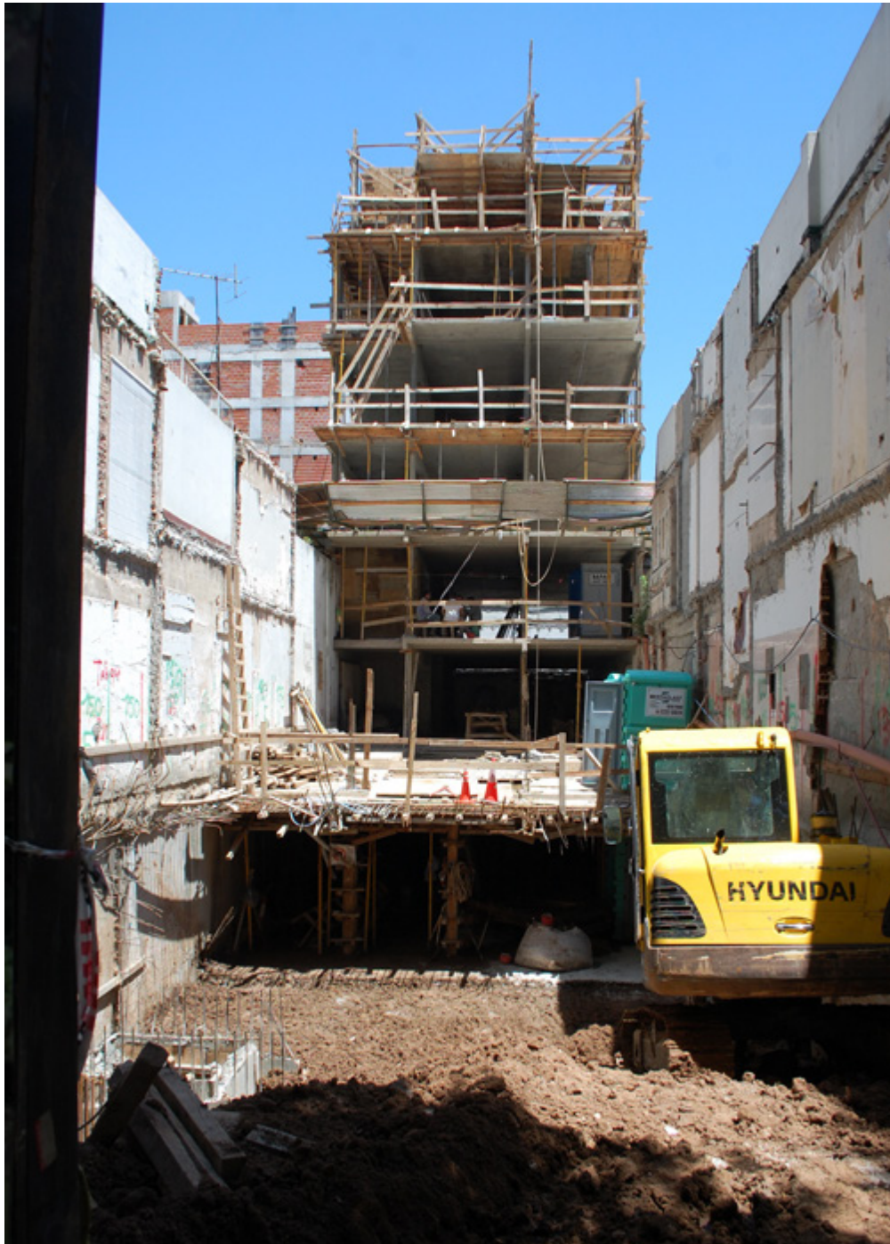
Reinforced Concrete Structure and Parking Excavation Modelle AdeF Building, Buenos Aires, Argentina
