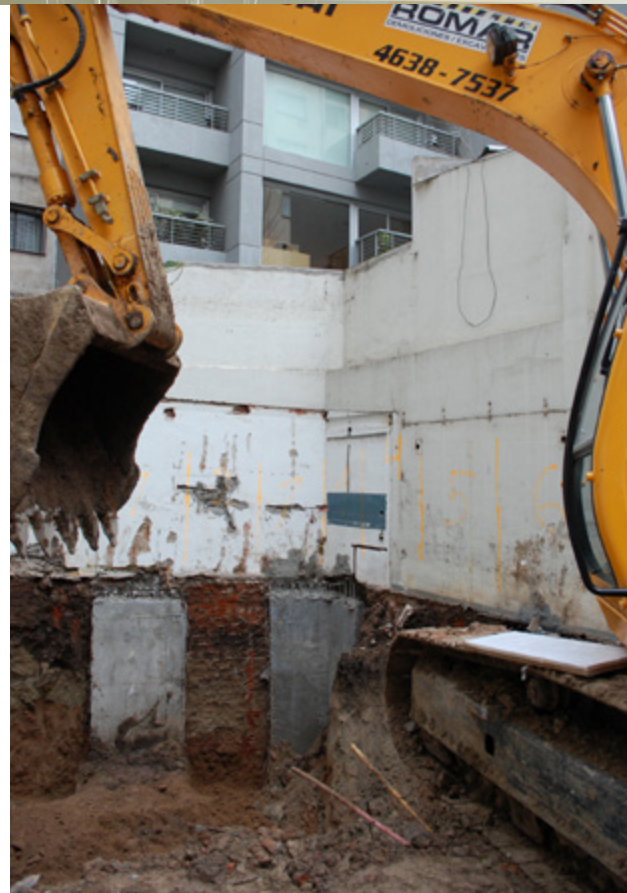
Foundation Excavation and Submersion Works, and Entrance Portico. Modelle Ocampo Building, Buenos Aires, Argentina
